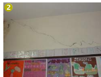
▲ Cracks in the walls, caused by the earthquake
